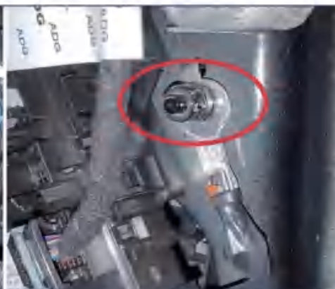
Negative cable connection
